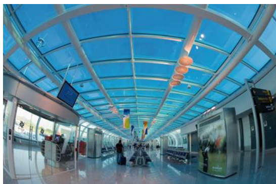
Brazíl: TROX swirl diffusers distribute fresh air to the halls and corridors of Rio de Janeiro's Santos Dumont Airport.
